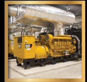
UNINTERRUPTED POWER SUPPLY
